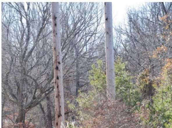
Figure I-5: Big Island-Reusens 69-kV Line Structure 432-16: Multiple Pole Cavities and Pole Splitting
