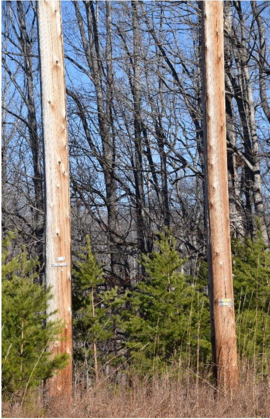
Figure I-7: Big Island-Reusens 69-kV Line Structure 432-18: Woodpecker Holes
